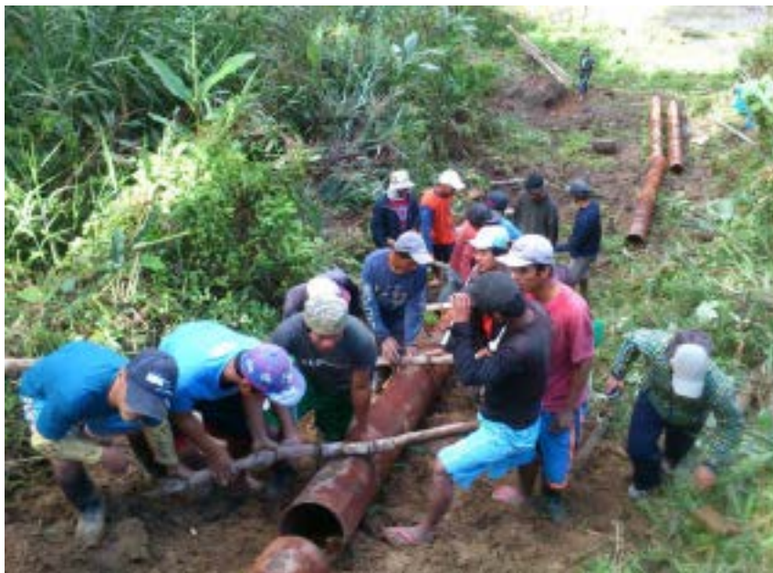
Figure 3. Community volunteers from Parina MHP hauling a steel penstock in ‘bayanihan’ fashion. (Photograph courtesy of DLSU.)
