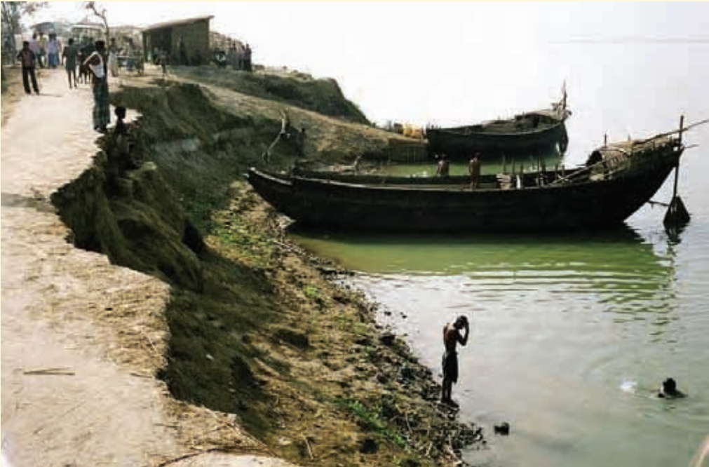
A collapsing road in the Bengal Delta (photo: Professor Graham Chapman)
