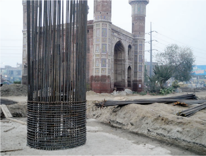
Figure 14. View of the Orange Line's viaduct foundation beside the Chauburji Gateway in Lahore, Pakistan. (Image: Durham UNESCO Chair).
