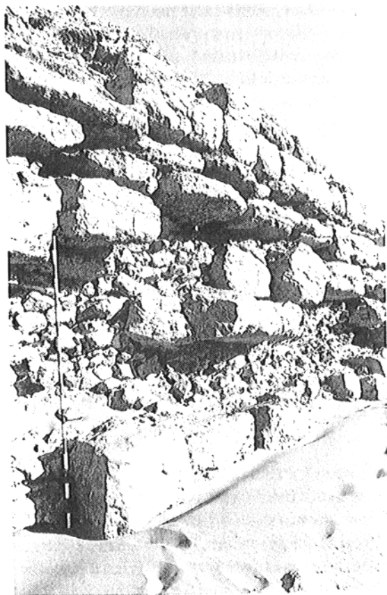
Figure 6. View of the western face of the breakwater showing how it was built, with an interior core of concrete faced by limestone blocks.
